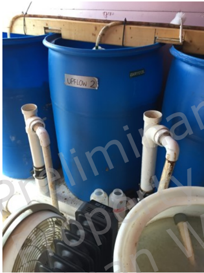
On-ground denitrifying bioreactor
