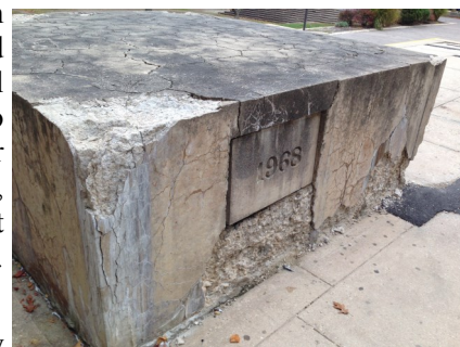
Up close, the exterior of the building is showing its age.
