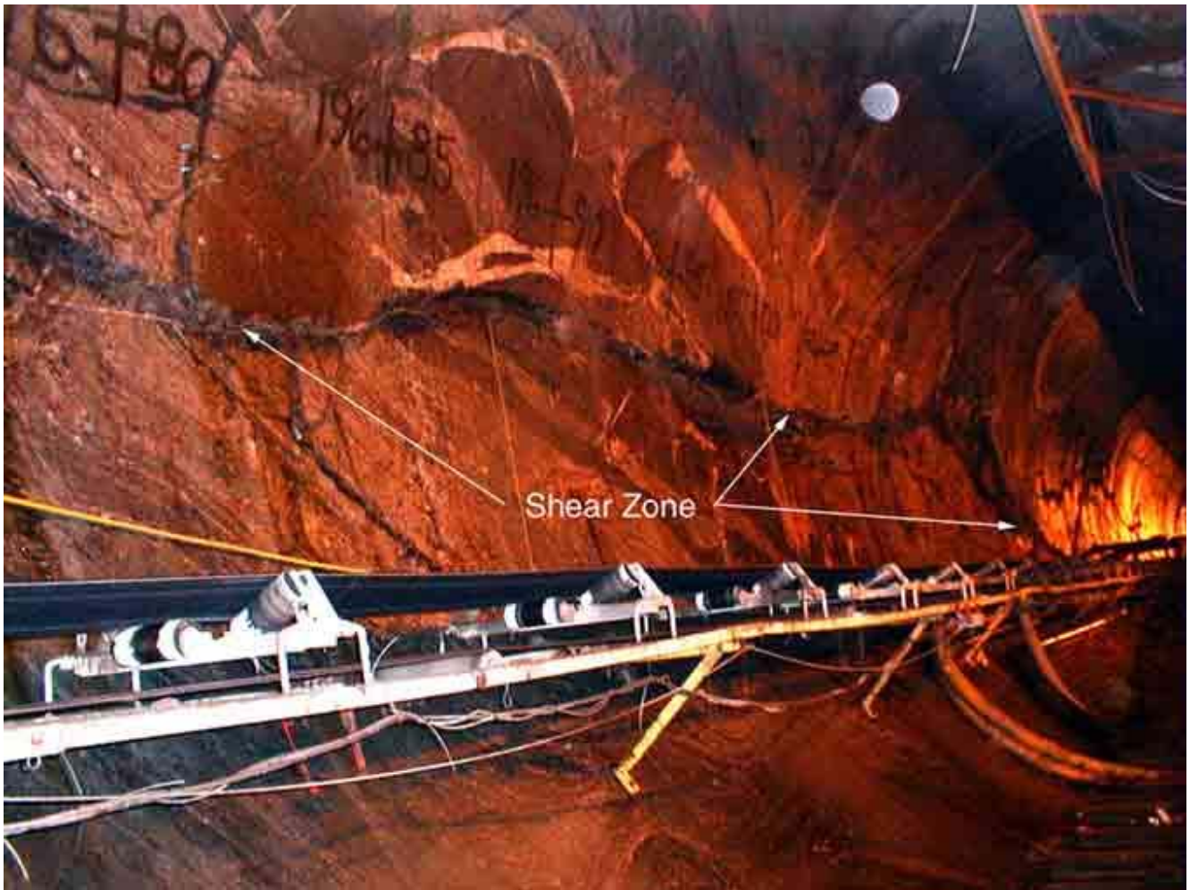
Figure 4 – View of migmatitic amphibolite, dioritic gneiss, and minor biotite schist highly fractured because of composite movement along a SW-dipping shear zone. The shear zone is a continuous gently dipping feature for 107 m that originates at Station 195+25 and continues on both tunnel walls to Station 198+50. Here it steepens and disappears into the crown of the tunnel in a zone of ramping imbricate fault splays. Fault gouge and -breccia vary in thickness from 0.4m thick in areas of fault splay intersection near the central reach of the zone to a hairline fracture at the end. [Image by C. Merguerian, 18 November 1999.]
