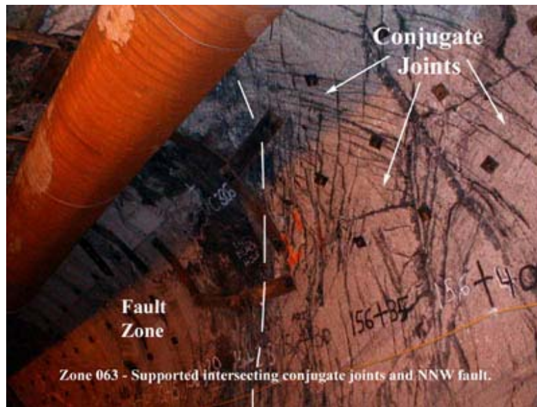
Figure 9 – Left wall view of a N20°W fault of Group E that cuts invert at 156+35 with a 0.5 to 1.0 m thick crush breccia and adjacent area of intersecting conjugate joints (flower structure). [Image by C. Merguerian, 30 December 1998.]
